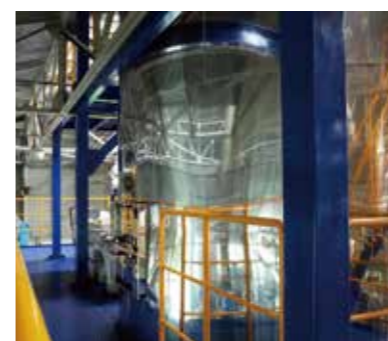
Atomization mode: Rotary atomizer Drying chamber diameter: φ3400 mm Water evaporation capacity: 86 kg/h
